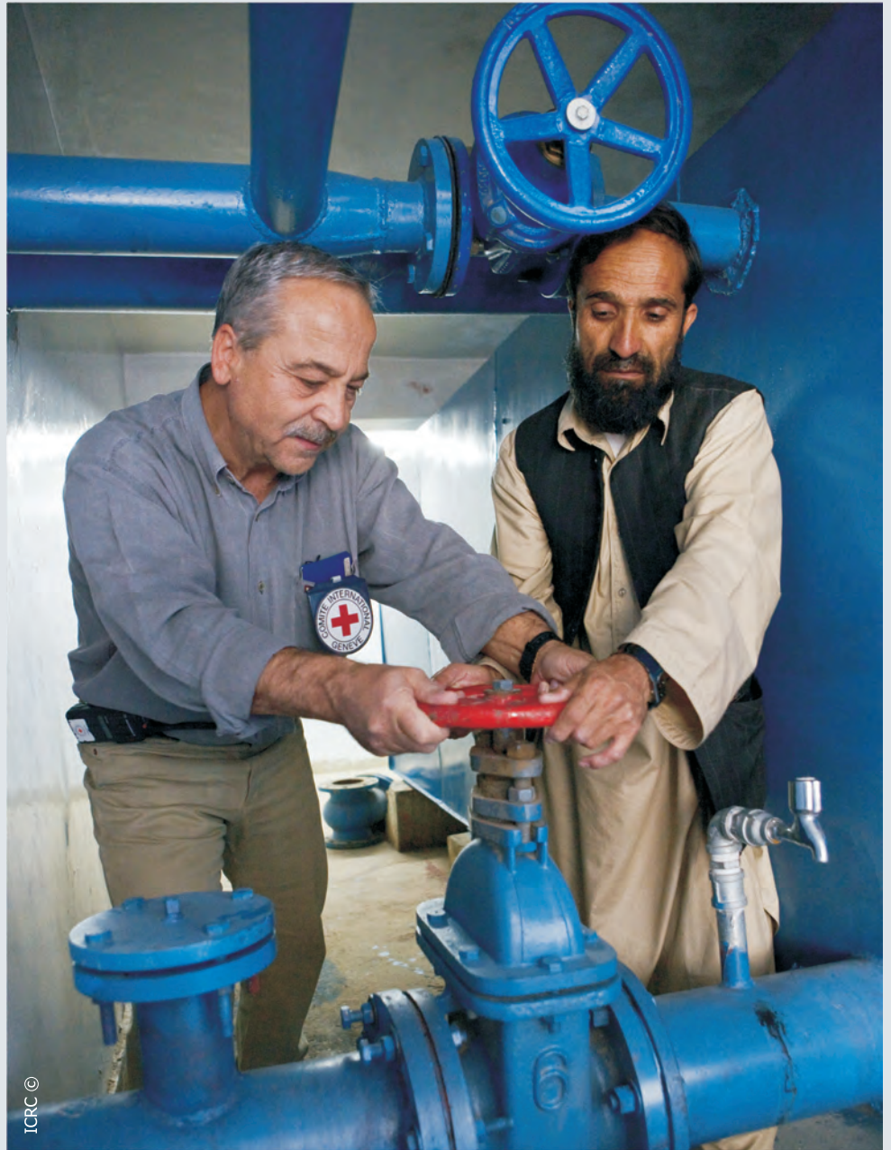
The ICRC rebuilt the water tank in Mirwais regional hospital which provides water to the entire hospital facility, Kandahar
