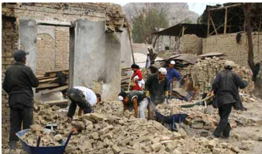
More than 2'800 daily workers, most of whom came from the areas directly affected by the violence, participated in a cash-for-work programme to clear rubble, ash and debris from the destroyed or burnt houses and surrounding streets. The wages received by the workers helped them to cover their basic needs and those of their families.
