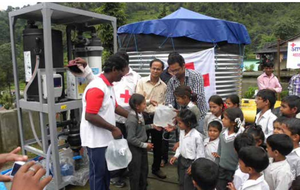
Red Cross and local community workers distributing water after installing the Water Purification Unit in Phata, Rudraprayag
