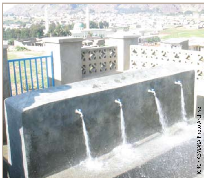
Solar-powered water supply system built by the ICRC, Aklelet, Gash – Barka region.
