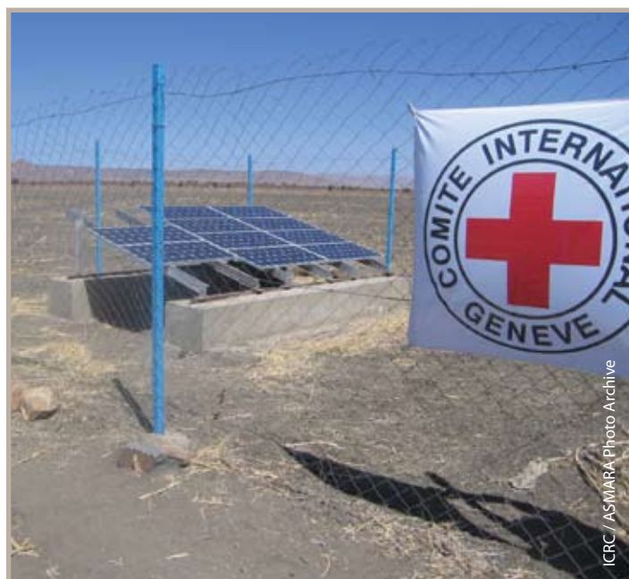
Solar-powered water supply system built by the ICRC, Berik Hutsa, Debub Region.
