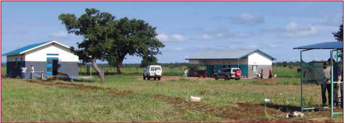
Rehabilitation and construction of maternity ward at Omot health centre in Pader district
